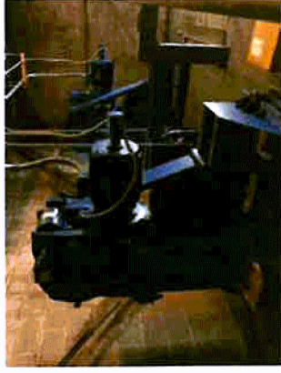
88 : Traction elevator machines
