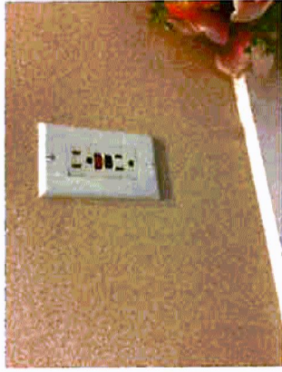
86 : Typical GFCI outlet in restroom
