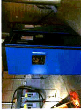
87 : Traction elevator controls in the mechanical penthouse
